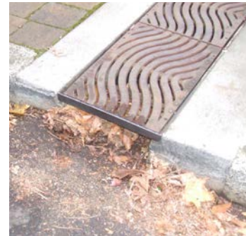
Clogged water access
