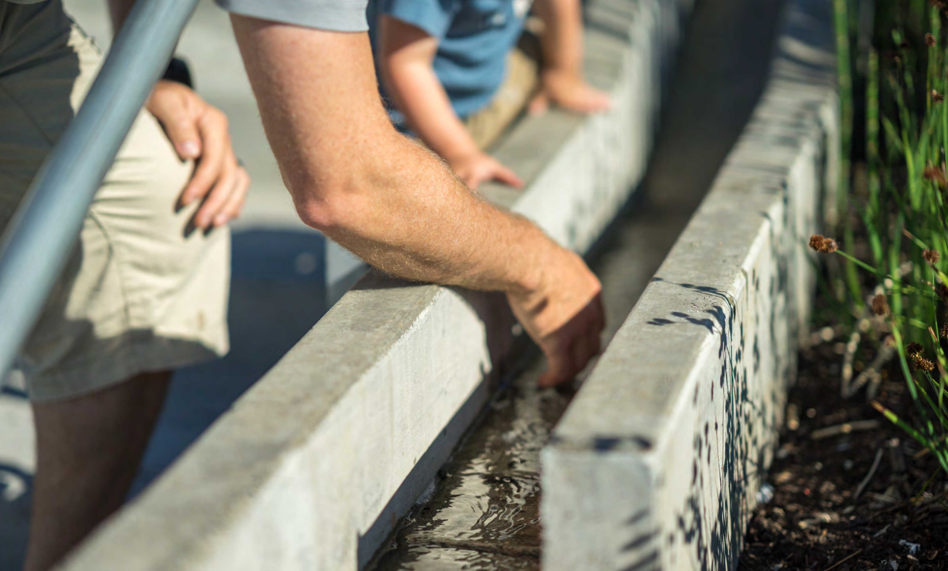
The storm water runnel collects run-off in and around the Hillclimb and conveys it along the stair.
